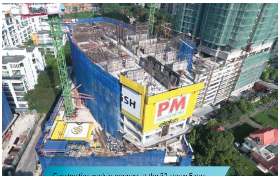
Construction work in progress at the 52-storey Eaton Residences at Jalan Kia Peng, Kuala Lumpur
