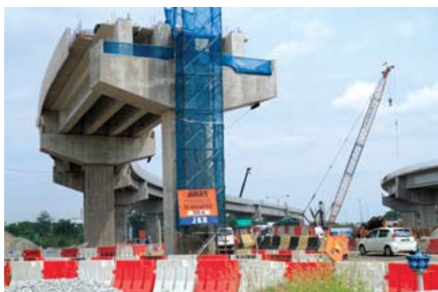
Design and build project for a bridge across the railway at Jalan Pelabuhan, Port Klang, Selangor.
